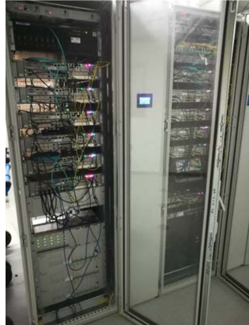
FAIR Ring BPM test bench installation
