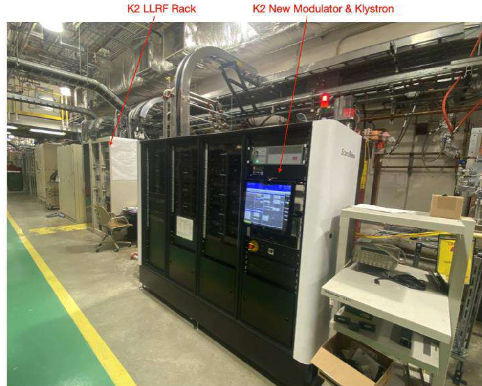
New K2 modulator, klystron and LLRF racks in Linac Gallery
