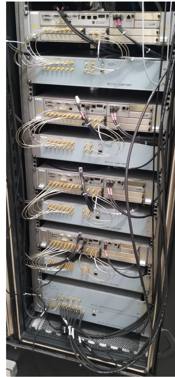
One of the four LLRF racks in DIS during pre-installation SAT period
