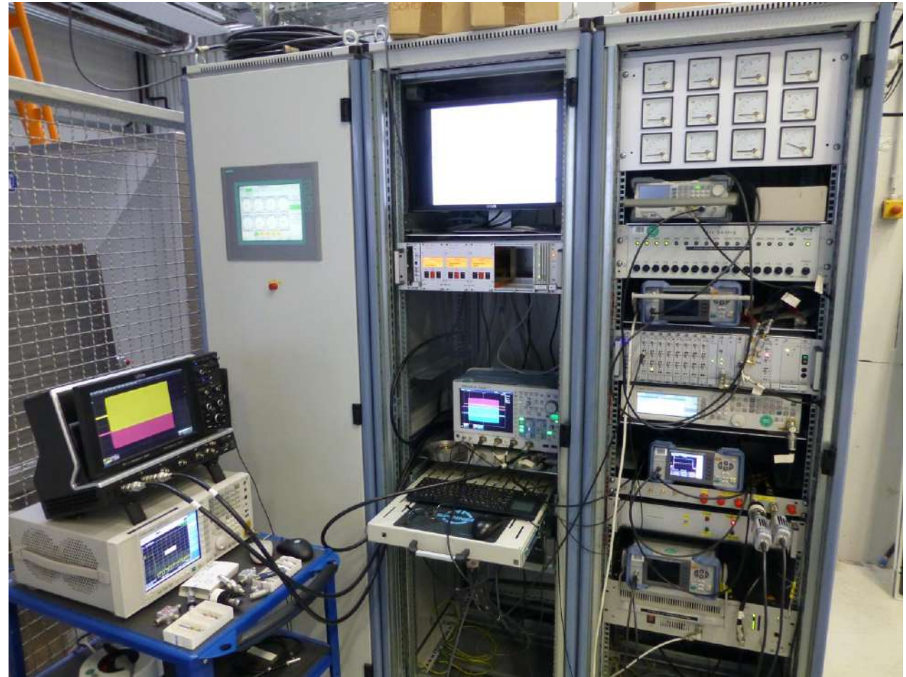
Resonant Frequency Control with stepper motor controllers, ARC detection system, fast interlock system and measurement, master oscillator, power meters and 300 W klystron driver
